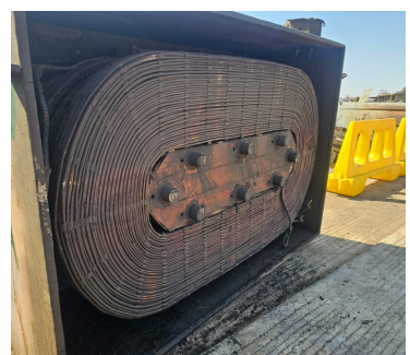
MAGNET WINDING EXPOSED
